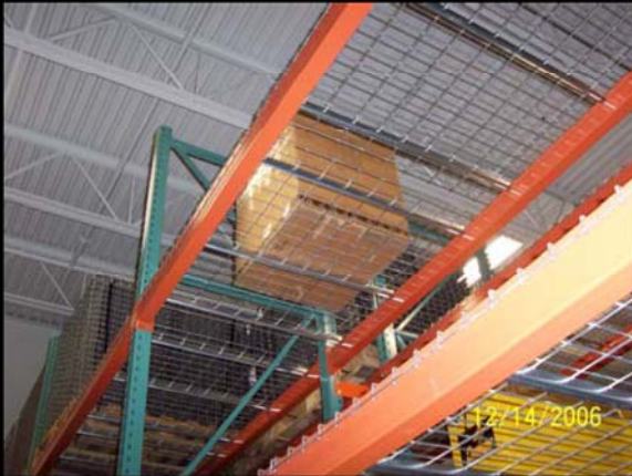
POINT LOADING: NOT ACCEPTABLE FOR USE OF WIRE DECKING. NOTE THE MATERIAL IS SUPPORTED ONLY BY THE WIRE DECK
